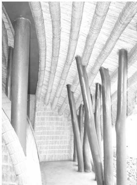
Image 2.2: ‘Inner rings’ of the roof of the main building of the Royal Kasubi Tombs, reeds tied with sisal rope.
