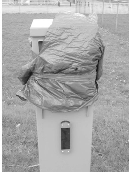
Figure 29: Broken intercom at the Terneuzen control room.
