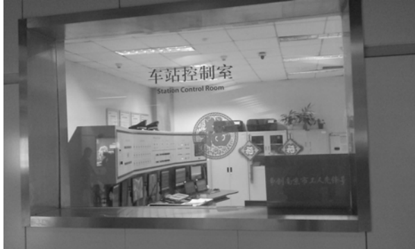
Figure 5: 2016 photo of an underground control room in Shanghai, visible to the public through a window, with text in (both Mandarin and) English: "Station Control Room". For several years there was a similar control room at Berlin's Alexanderplatz underground station, where you could speak directly to the BVG operator through a circular window. Sometime in 2019, an updated version of the control room was closed.
