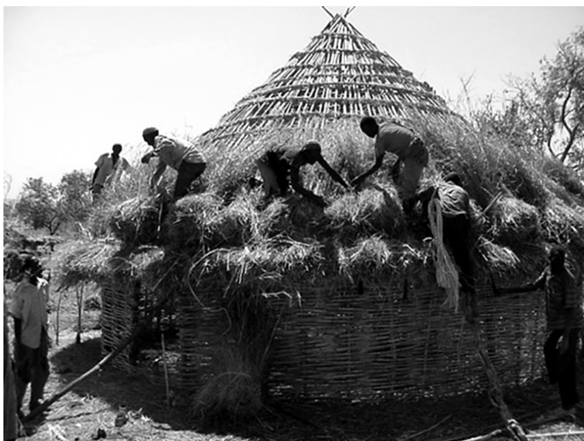
Fig. 6: Thatching a house through the amaha . Keshaf (Khomosha wereda).
