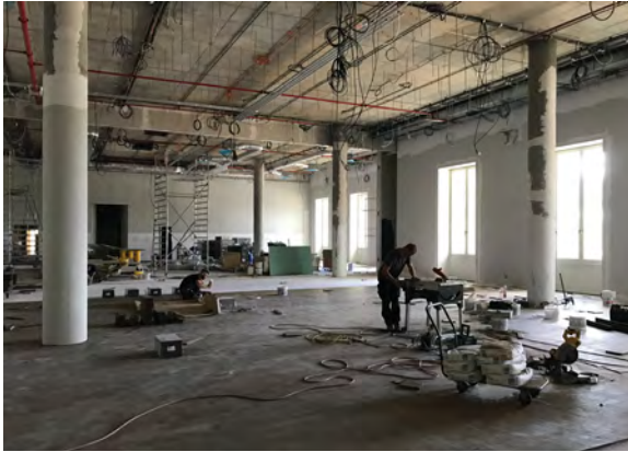
Shell construction stage of the exhibition spaces of the Humboldt Lab, May 2019. © Friedrich von Bose
