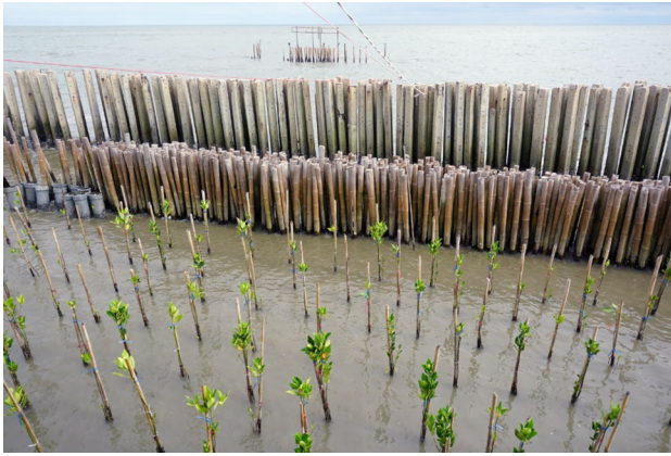
Figure 5: Coastal protection measures in Bang Khun Thian.
