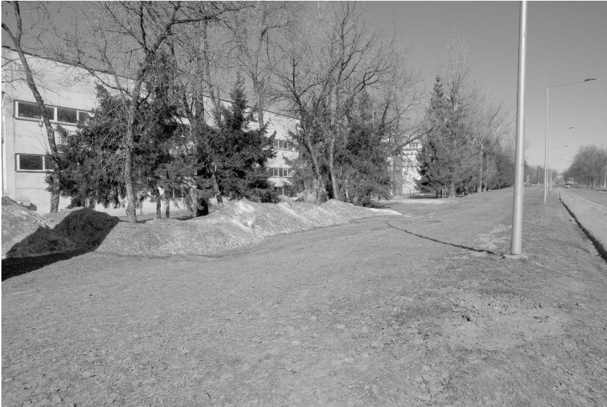
Figure 10. Revisiting one of the digging sites, where the soil was evened out and the cables were already covered with soil and thus invisible.
