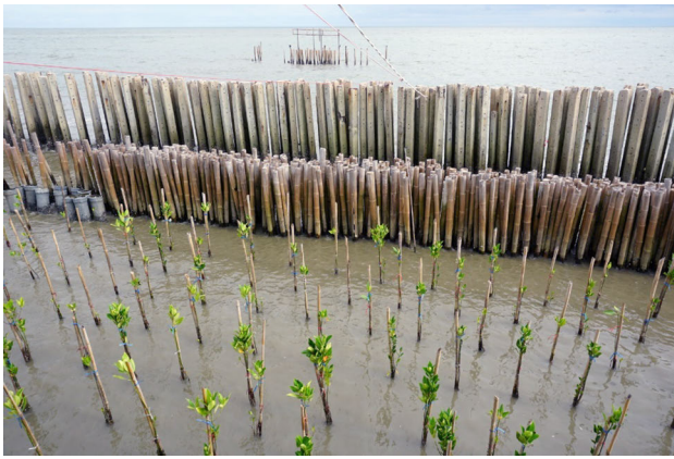
Figure 5: Coastal protection measures in Bang Khun Thian.
