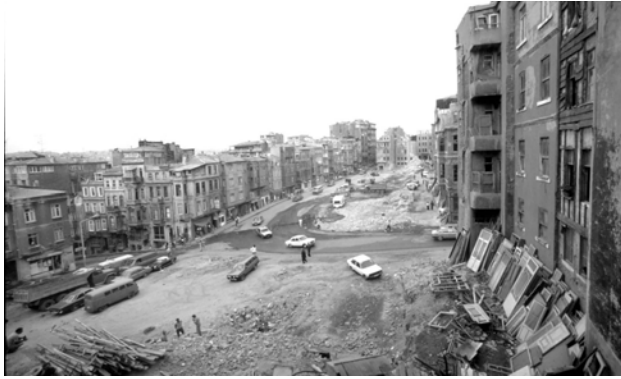
Figure 4.9: A general view of the demolition and salvage activity in Tarlabası. On the right, reclaimed doors are leaning on the buildings. On the left, there is a heap of wood
