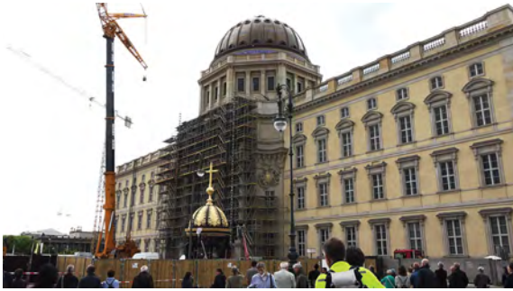
New cross and lantern before installation on the dome of the Humboldt Forum, Berlin, May 29, 2020. © Tal Adler
