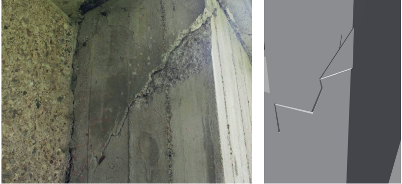
Figure 5.12: Representation of a spalling at the abutment.
