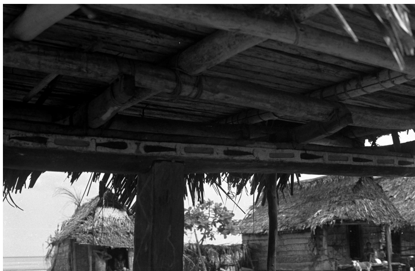
Fig. K7: Close-up of the joint where the vertical post ( kokola bwala ) carries the horizontal central canoe-shaped beam ( waga ). Note that both the post and the hole in the waga are square, preventing any rotation of the roof ( katua ) of this bomiyoyeva , of its floor ( bomakau ) or canoe-shaped beam.
