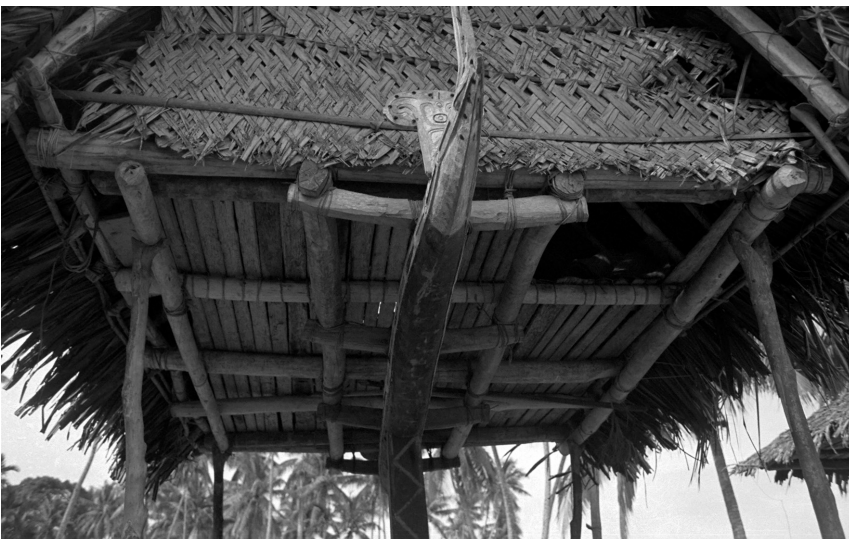
Fig. K5: Right rear side view. The horizontal beam ( waga ) is supported by the square central post ( kokola bwala ). The waga shows carved decorations ( tara-papa ) over its full length. The only access ( kaukweda ) to the loft ( tatom ) is just visible at the proximal corner of the building.
