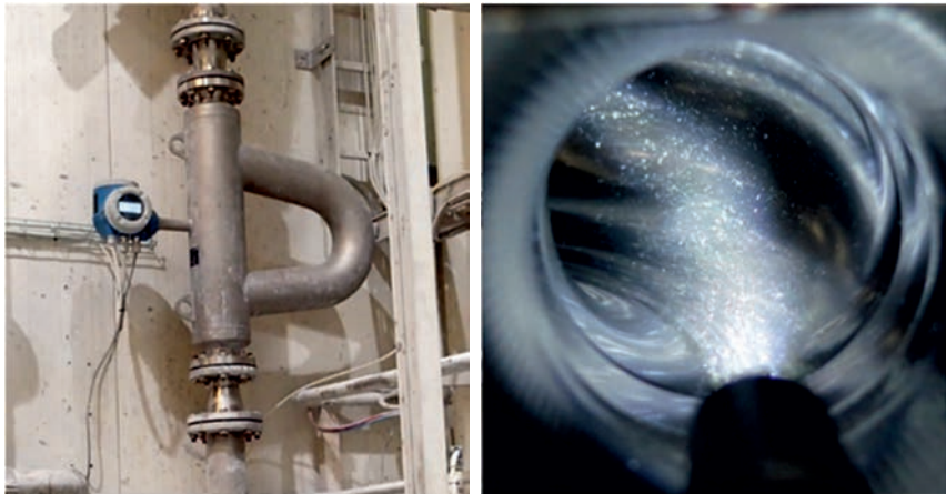
Fig. 6: Left: The installed Promass Q Coriolis flowmeter. Right: Optical investigation of the interior of one of the flowmeter's measuring tubes after 11 months in operation shows clear signs of abrasion.
