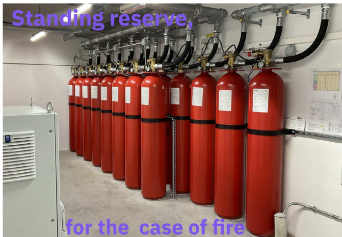
Fig. 4: The physical poster as part of the augmented reality data centre experience showing the gas cylinders from the university data centre »standing reserve, for the case of fire«
