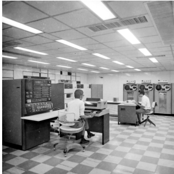
Fig. 3: The IIT Madras Computer Center with the IBM 370 mainframe computer after the opening in 1973. Photographed by Cadambi Gourishankar (Photo: Heritage Centre, IIT Madras).
