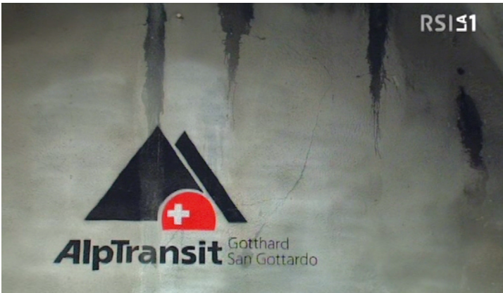
Fig. 37: Over the stencil on the last stone wall, first cracks appear.
