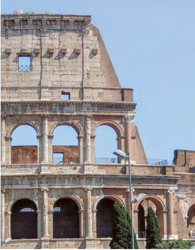
Fig. 2: Colosseum Rome – Giuseppe Valadier’s arch buttress repeating the original forms of the monument, photo 2021.
