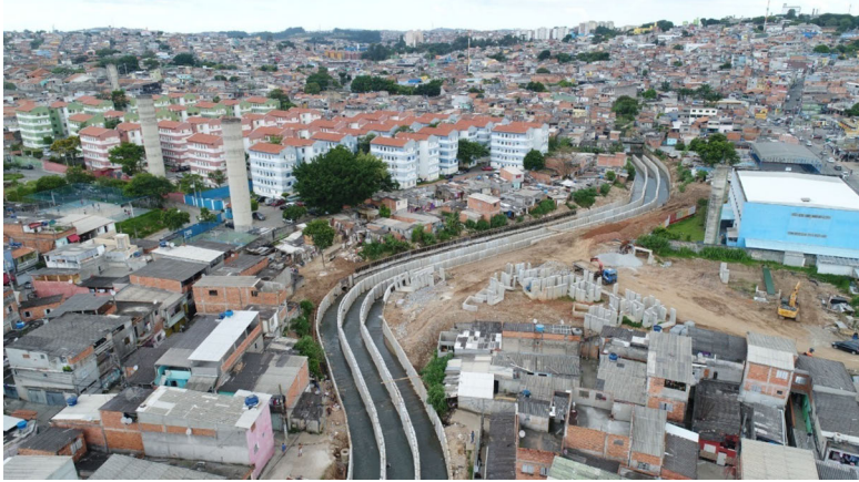
Figure 4: The Lageado stream emergency channelization works; infrastructure work on the canal, consisting of three culverts.
