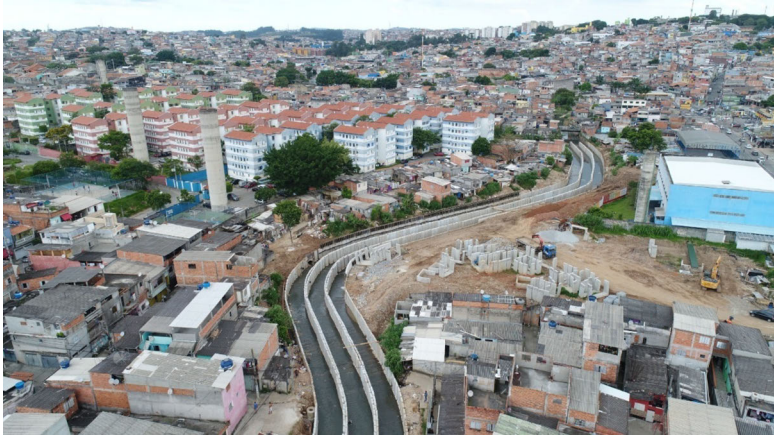
Figure 4: The Lageado stream emergency channelization works; infrastructure work on the canal, consisting of three culverts.
