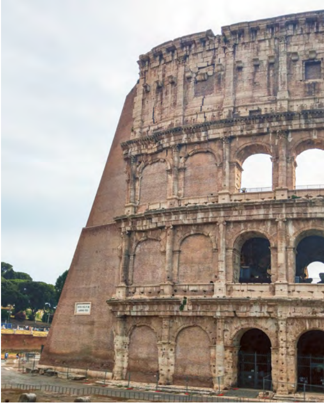
Fig. 1: Colosseum Rome – Raffaele Stern's reused brick buttress with the preservation of the appearance of crumbling arches, photo 2021.
