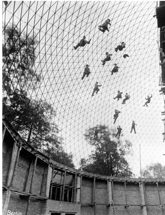
Fig. 2: Construction workers cling to the steel network of the Berlin planetarium under construction, early 1927. Courtesy Carl Zeiss Company Archives.
