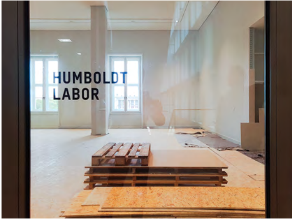
The Humboldt Lab inside the Humboldt Forum under construction, August 2020. © Tal Adler
